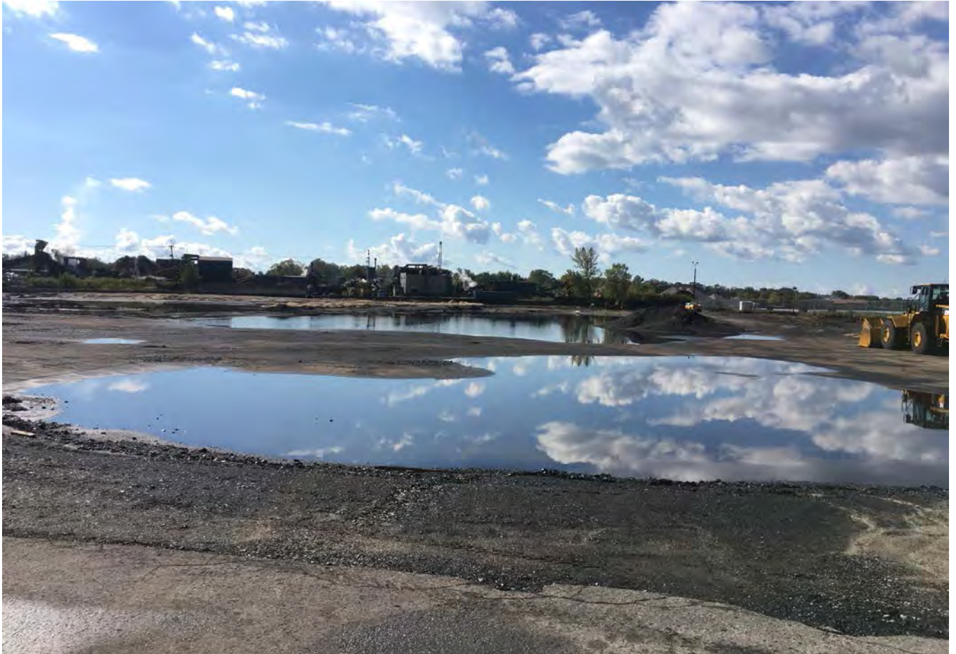
Flooding on site
