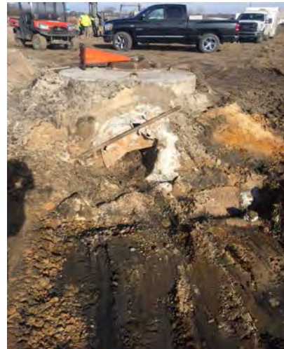
Drill MW-3 being installed (left) Preparation for the fantail at the stormwater manhole (right)
