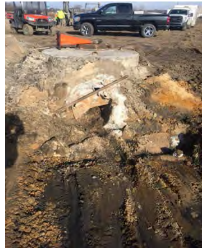
Drill MW-3 being installed (left) Preparation for the fantail at the stormwater manhole (right)
