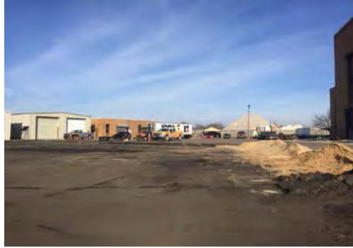
Cleaning of buried concrete pad. Sand added along parking lot/concrete pad dropoff
