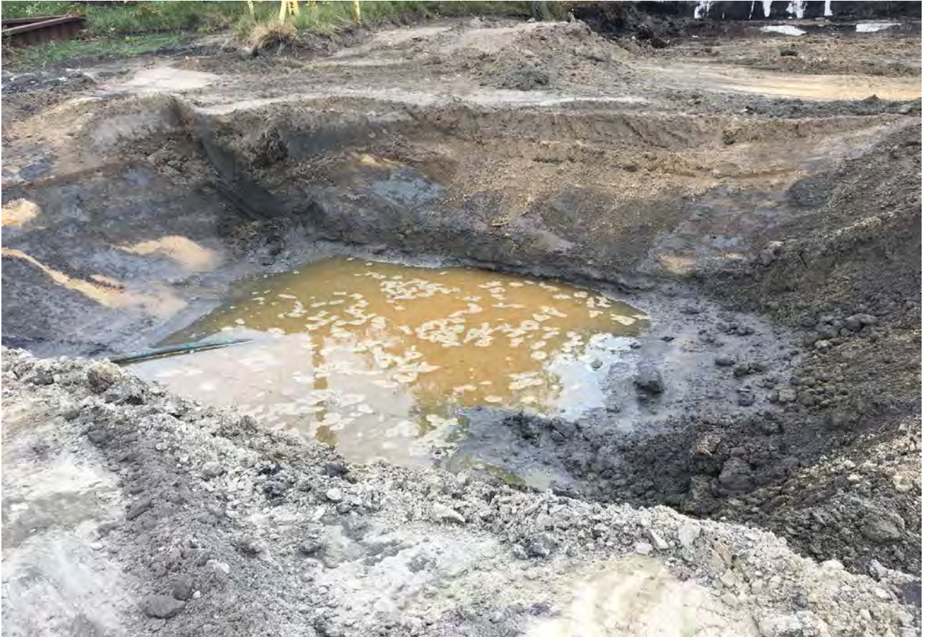
Area near south fence found to have CCR material and excavated
