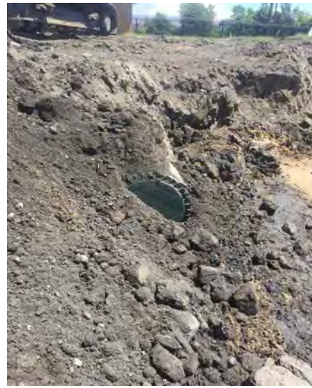
Cap on snowmelt line
