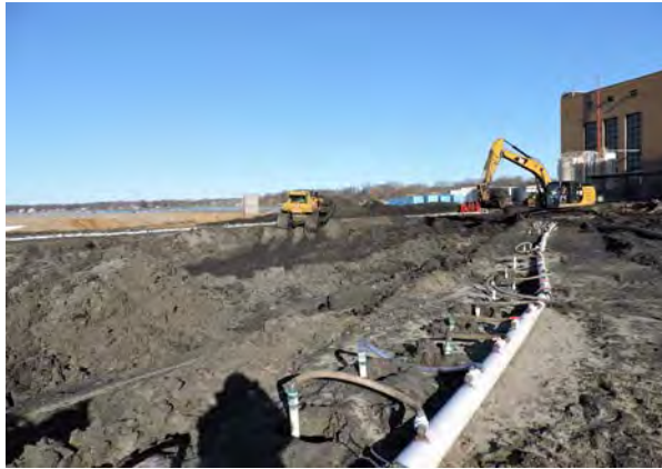
Ongoing excavation of CCR Area in the north portion of the CCR area
