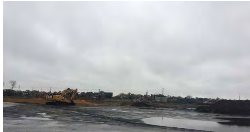
No construction activities past noon due to rain. Pictures of site from buried concrete
