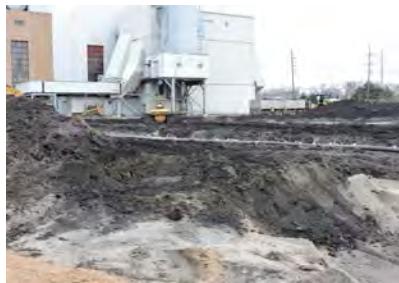
CCR material stockpile being loaded into the trucks to be taken off site
