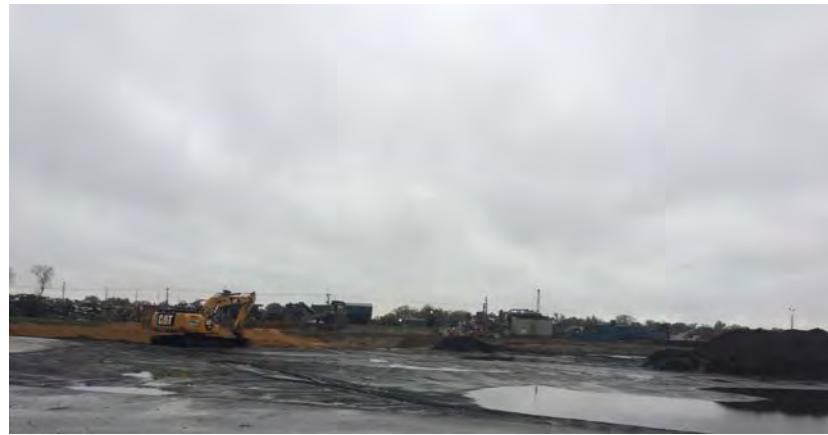
No construction activities past noon due to rain. Pictures of site from buried concrete
