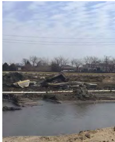
Pitsch Co. demo of the remaining concrete wall and weir near Pond 3
