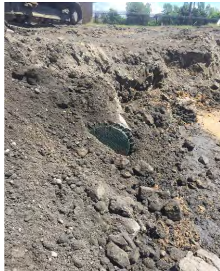
Cap on snowmelt line
