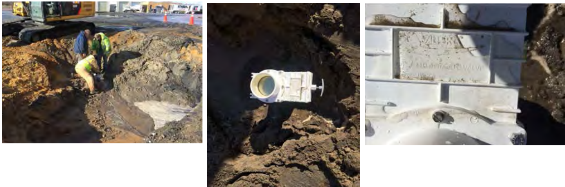
Gate Valve being placed on leaking storm pipe just east of the large concrete pad
