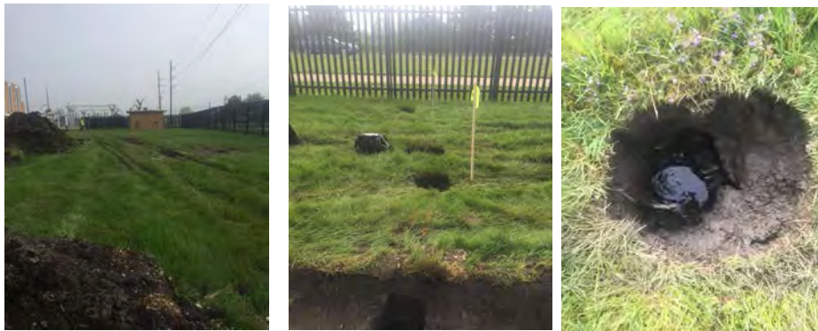
Holes over snowmelt lines
