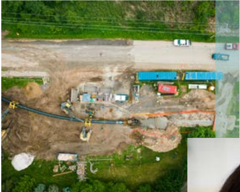
Photo courtesy of Prein & Newhof. Lakewood water main construction during the summer of 2022.
