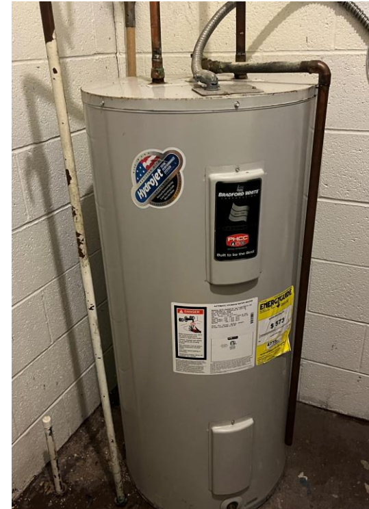
Uninsulated water heater pipes
