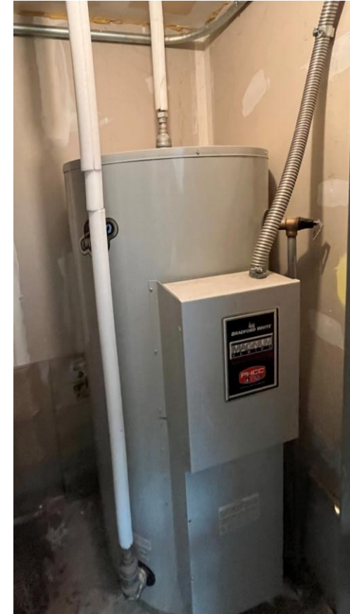
Insulated water heater pipes
