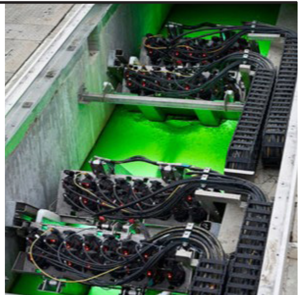
Example of a UV disinfection unit. Photo credit: Trojan.
